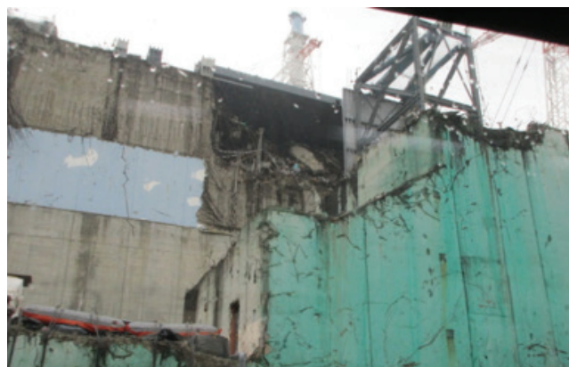
The upper side of the unit 3 reactor building at Fukushima Daiichi was damaged by a hydrogen explosion. This area housed the spent fuel pool and the fuel handling machines. (Courtesy: TEPCO)
